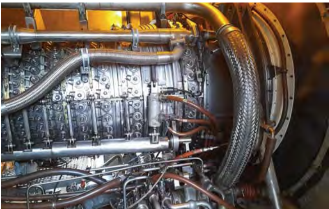
HPC General View R/H
