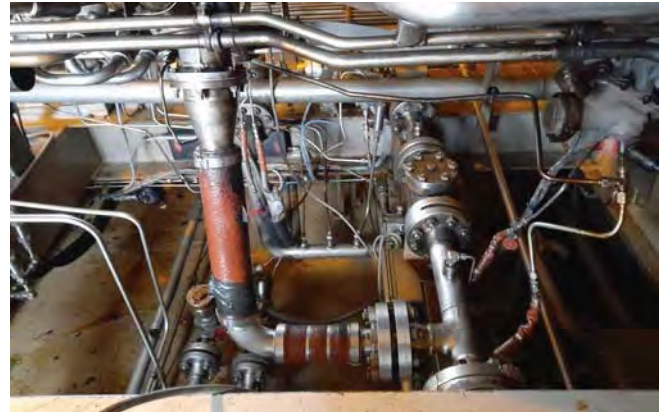
Gas Manifold and Piping's View
